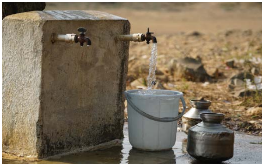
Figure 3C.12: Standposts in village
