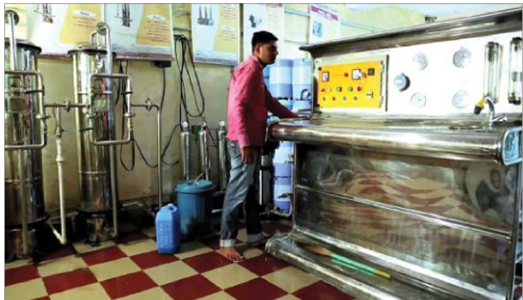
Picture 2.3: RO plant at Pansari, Gujarat
