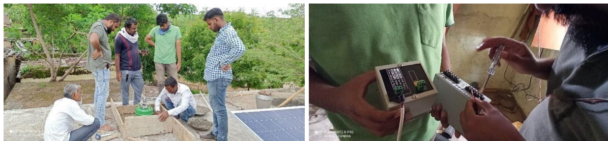
Figure 80 - Rain gauge installation at Gondala GP office
