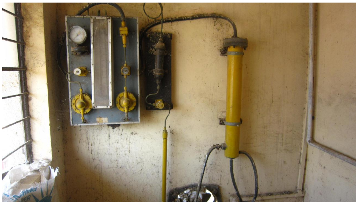
Figure 7.3 Dysfunctional equipment for adding chlorine to water
