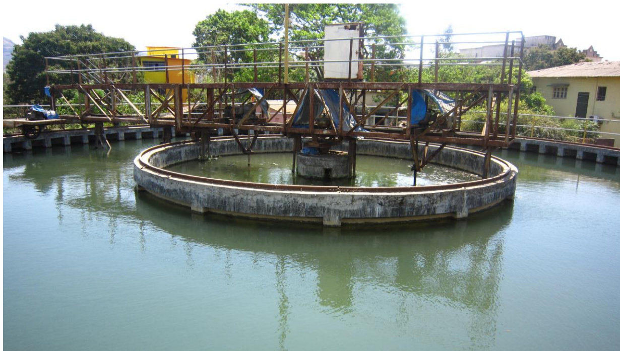
Figure 7.1 Water Treatment Plant at Dahivali. Karjat
